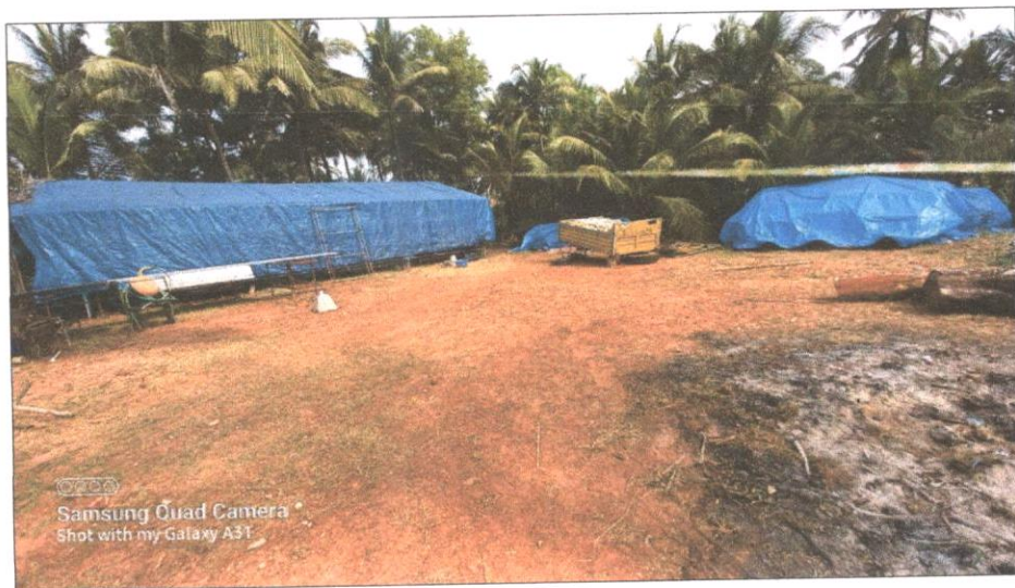
Pic 10: Temporary tent like structures (02 nos.) covered with plastic sheet (with some materials inside) were present at the site.
